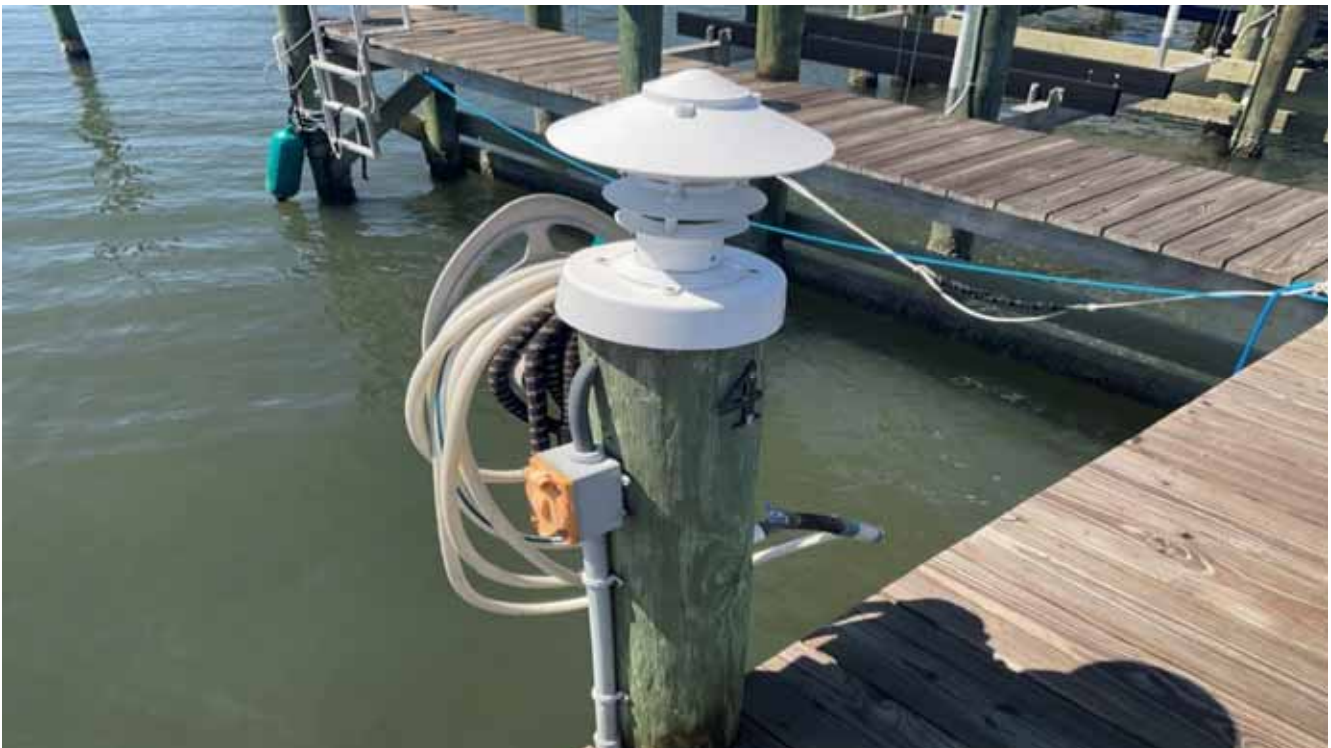
Boat Dock Electrical, Water
