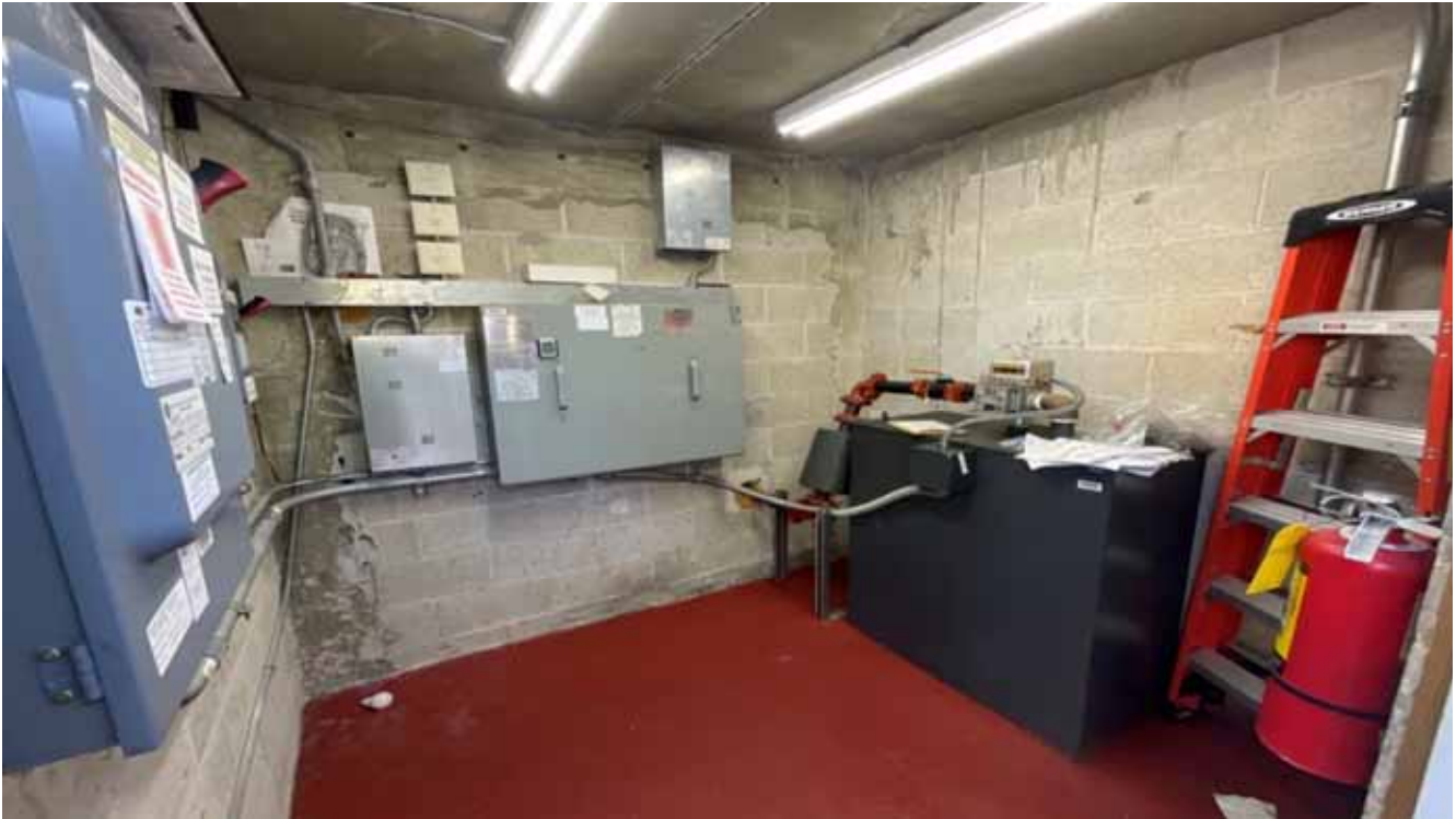
South Condo Bldg Elevator Equipment Rm
