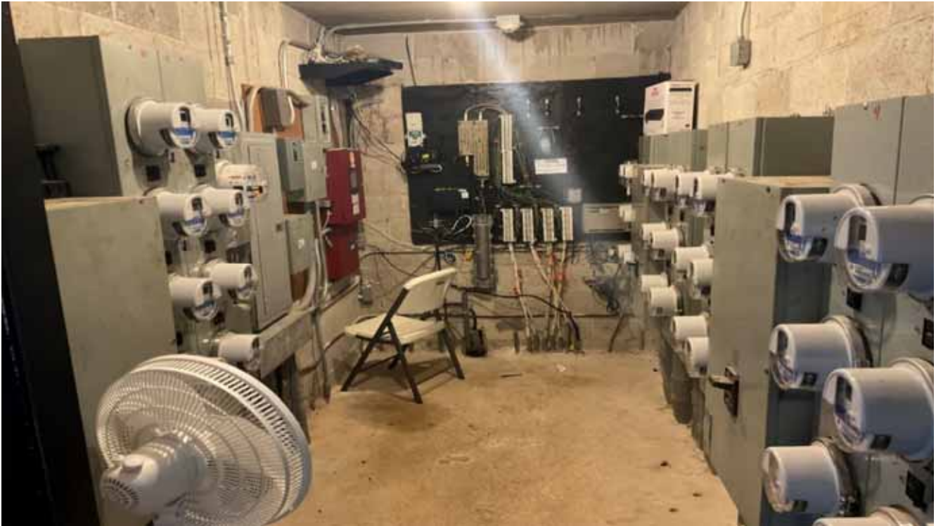
South Condo Bldg Electrical Rm
