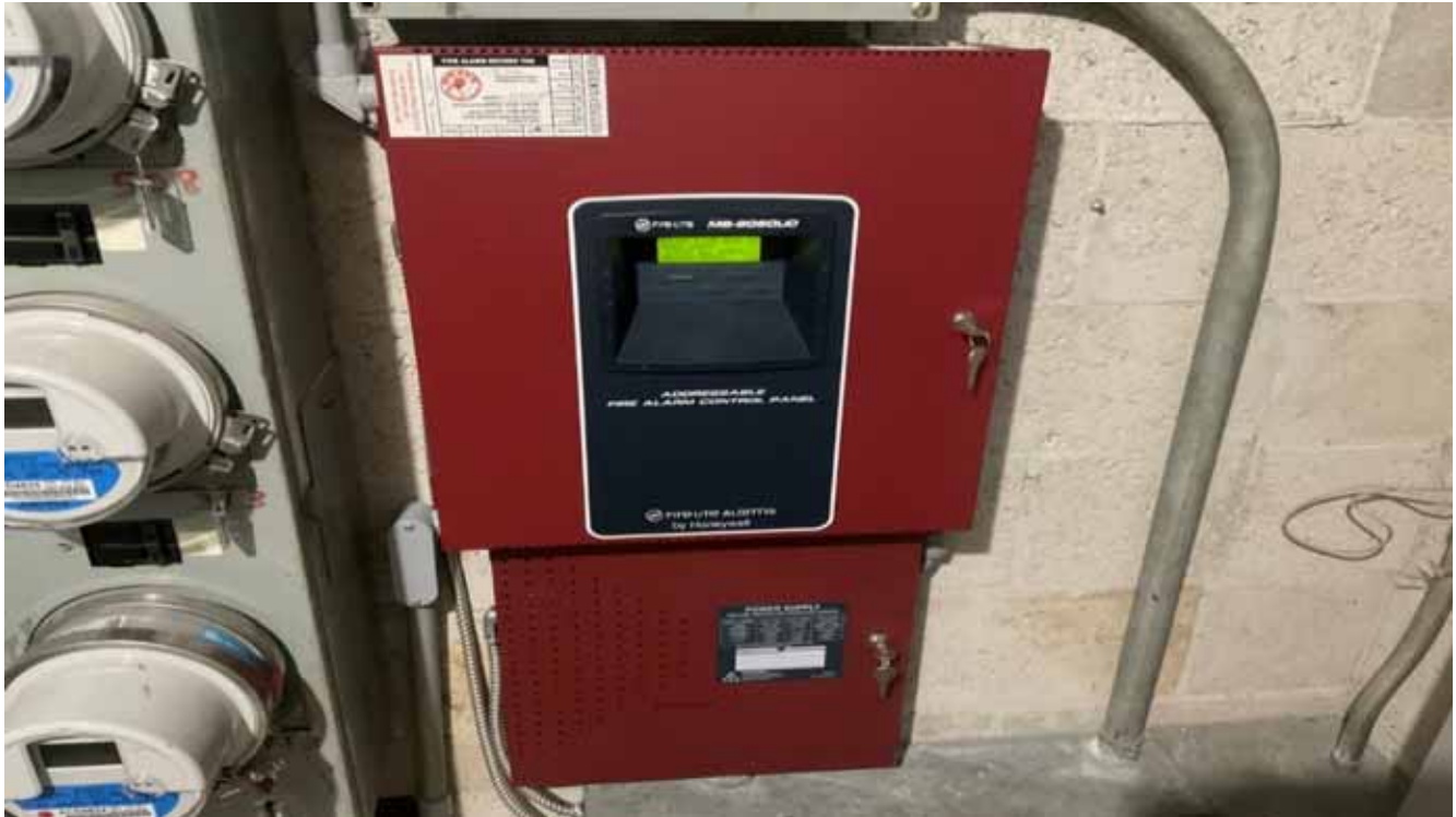
North Condo Bldg Fire Alarm Panel
