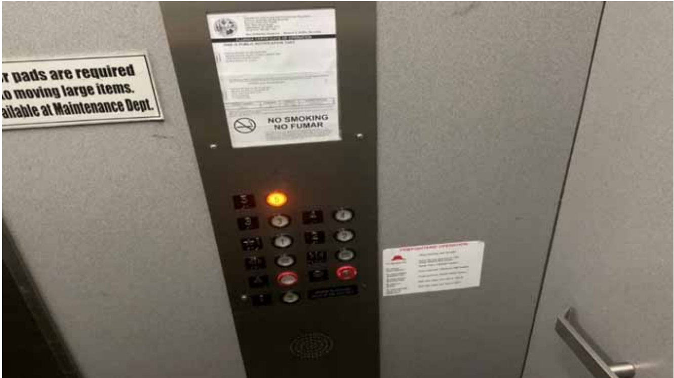
North Condo Bldg Elevator Cab
