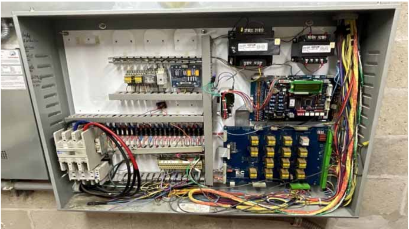
South Condo Bldg Elevator Equipment
