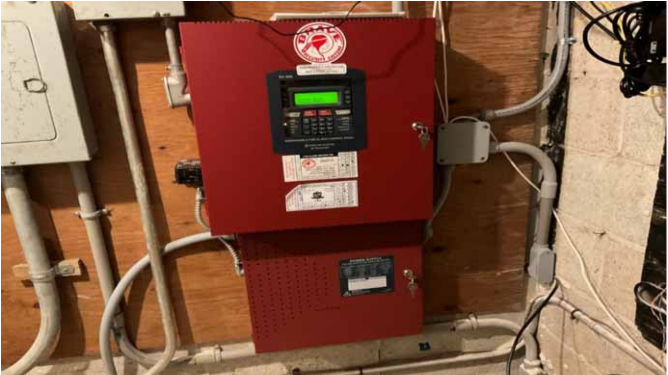
South Condo Bldg Fire Alarm Panel
