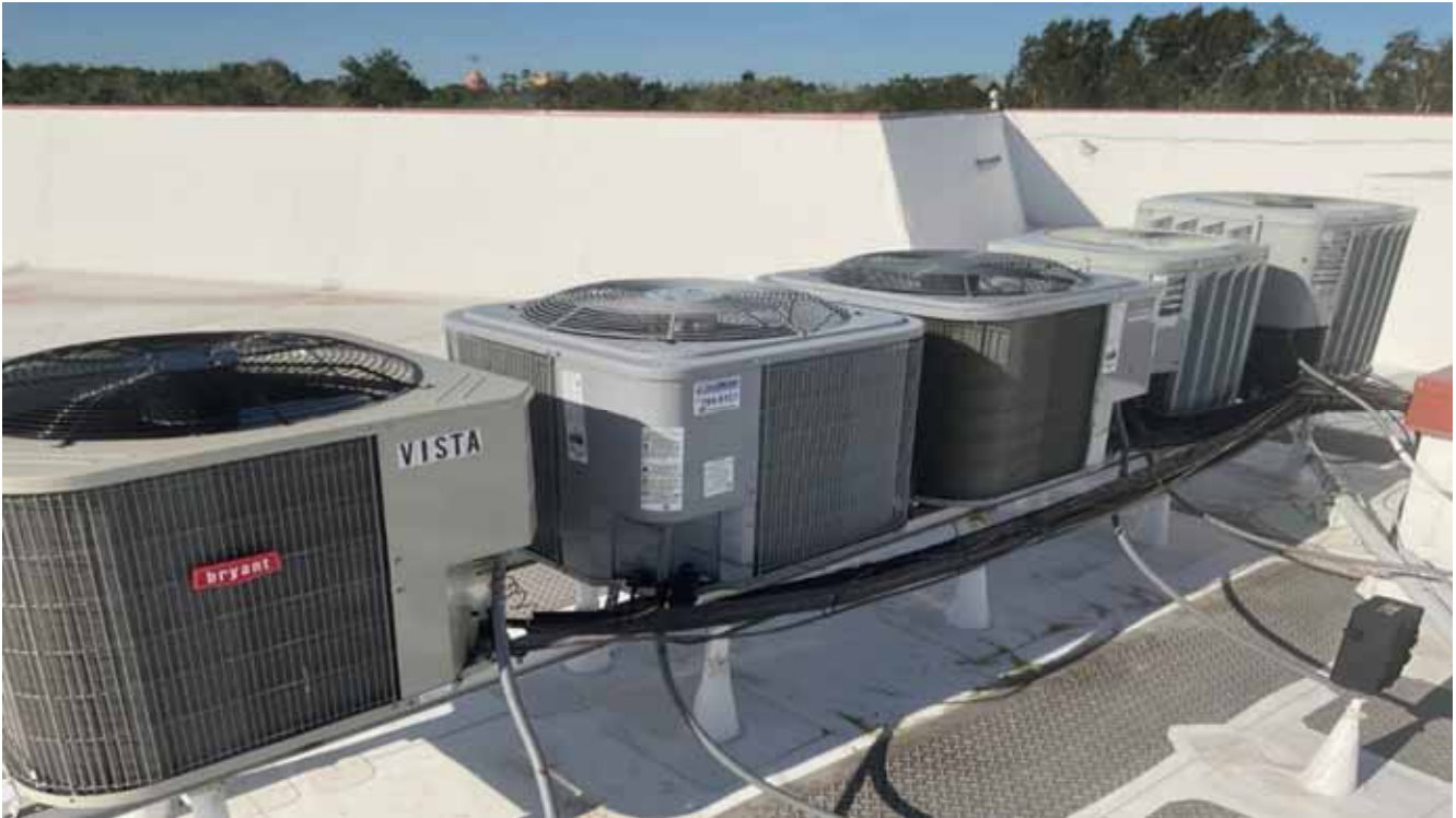
North Condo Bldg ACU's - Comm Area Rooms
