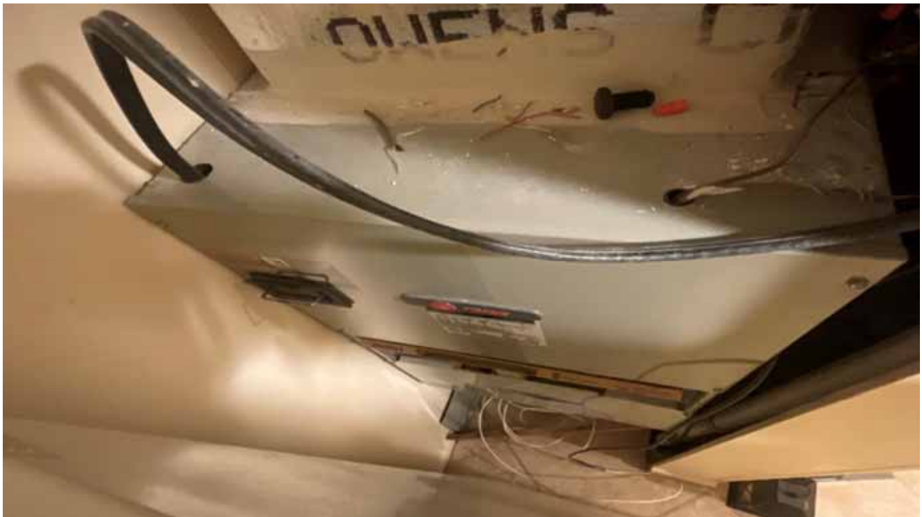
North Condo Bldg 2nd Floor River View Room AHU
