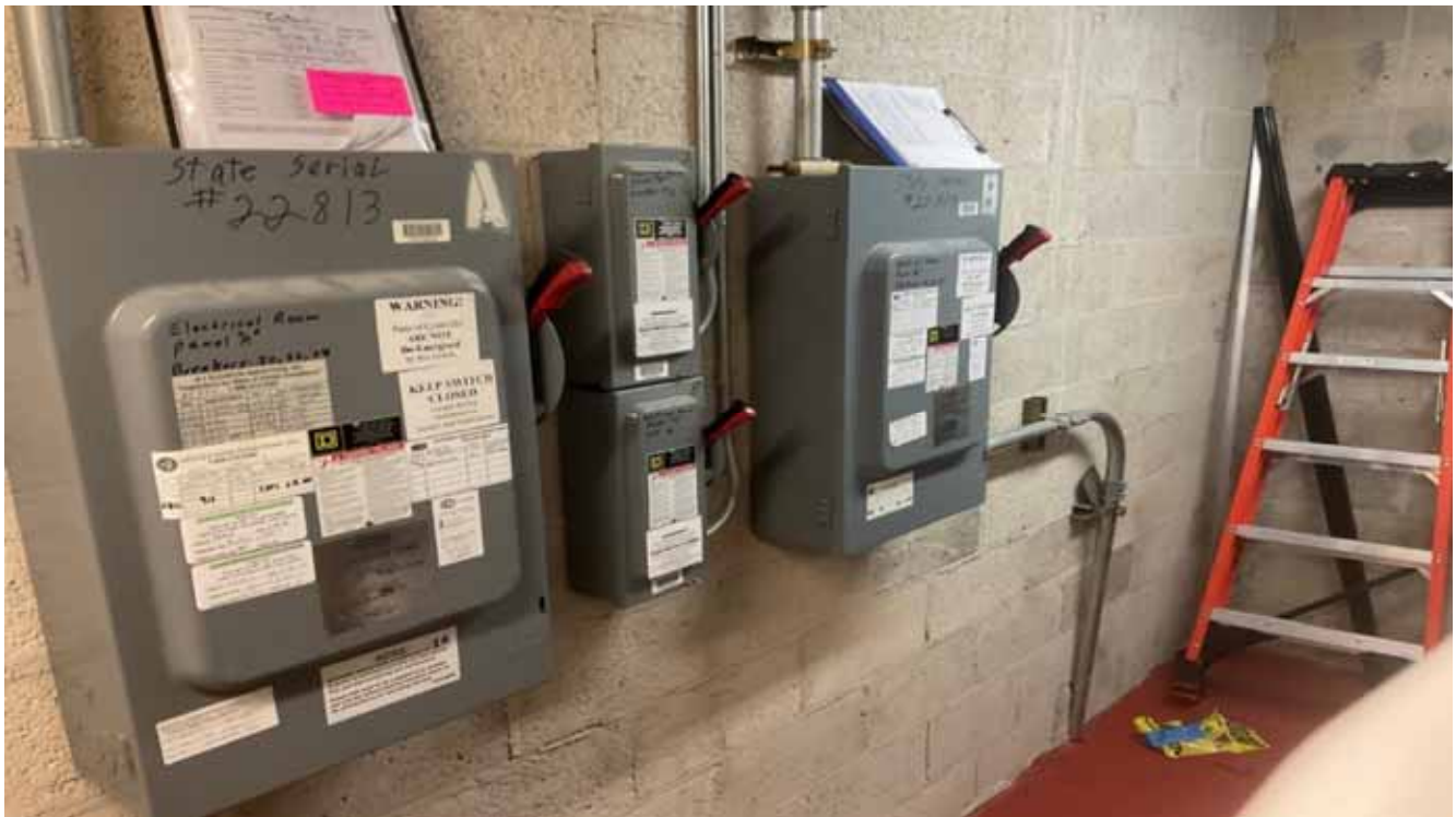
North Condo Bldg Elevator Electrical Panels
