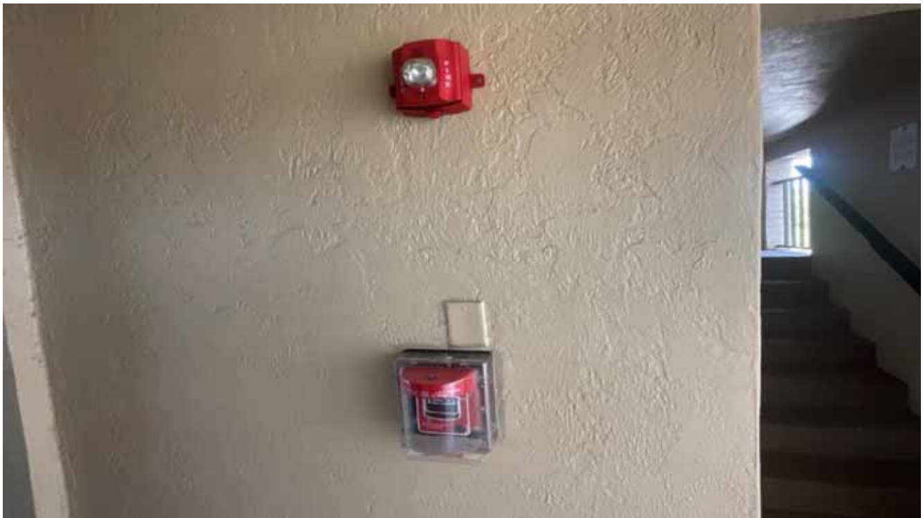
North Condo Bldg Fire Alarm System Devices
