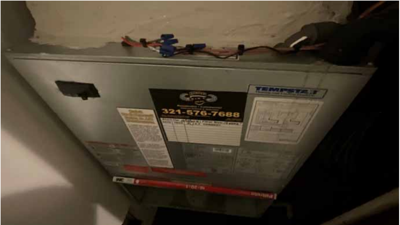
North Condo Bldg 3rd Floor Lagoon Lounge AHU
