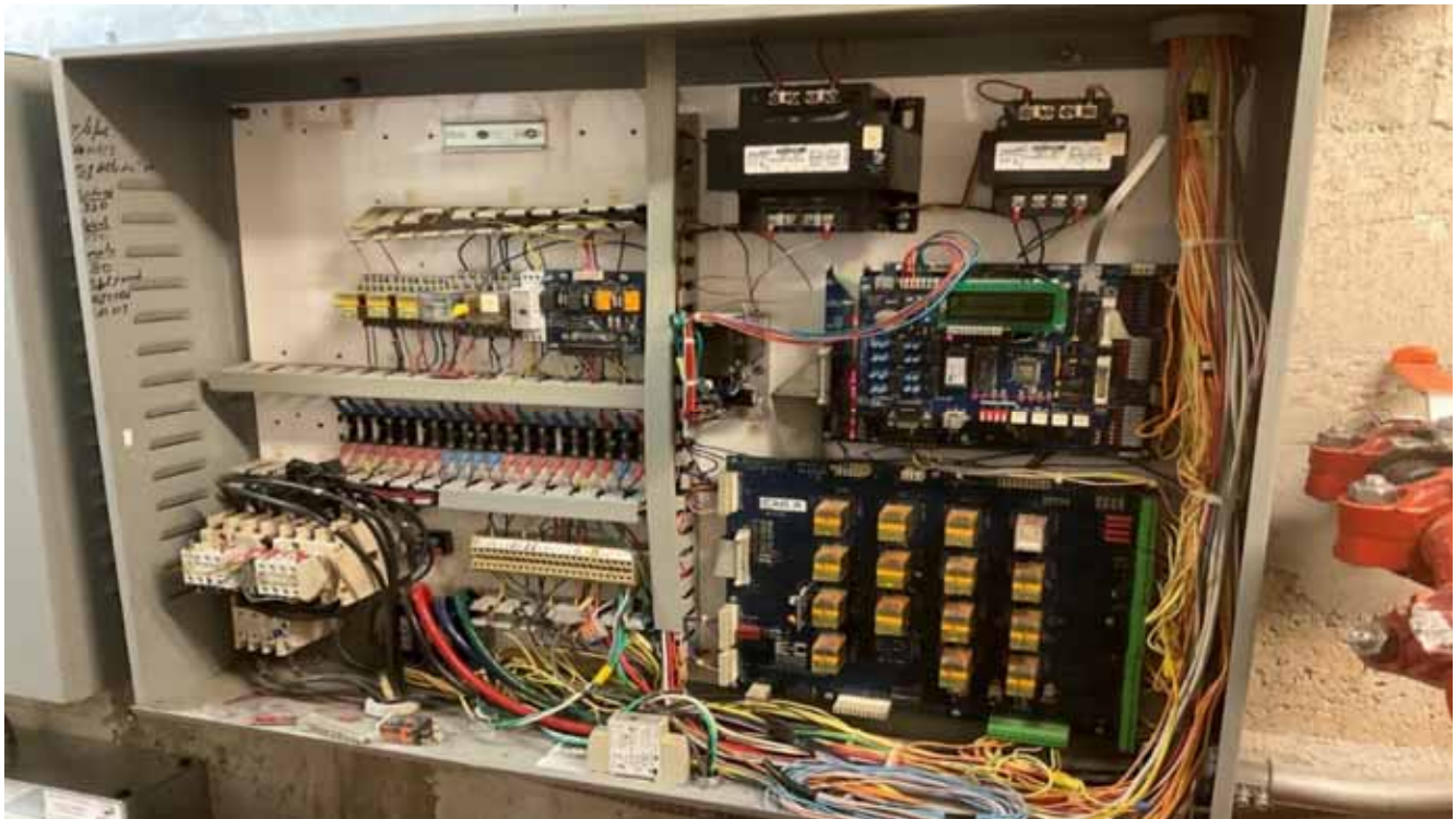
North Condo Bldg Elevator Equipment
