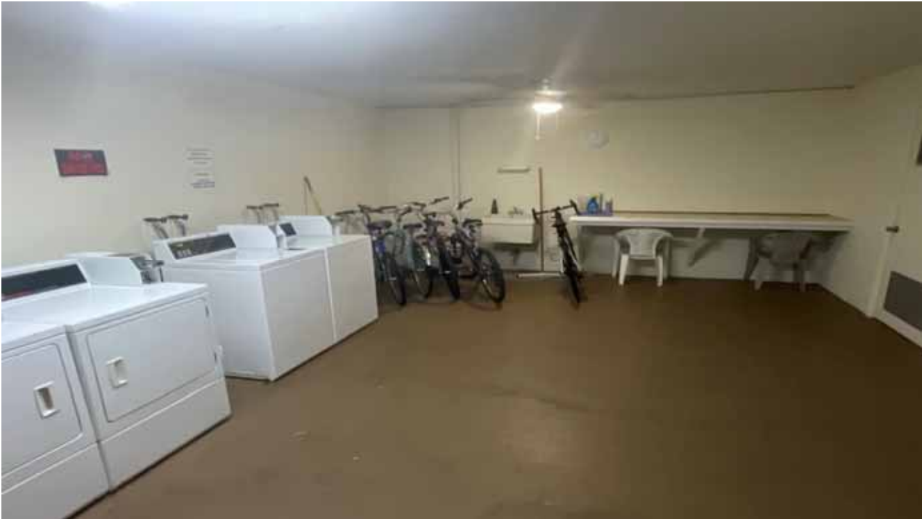
North Condo Bldg Laundry Room (Typical)
