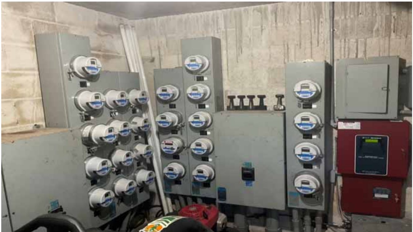
North Condo Bldg Electrical Panels
