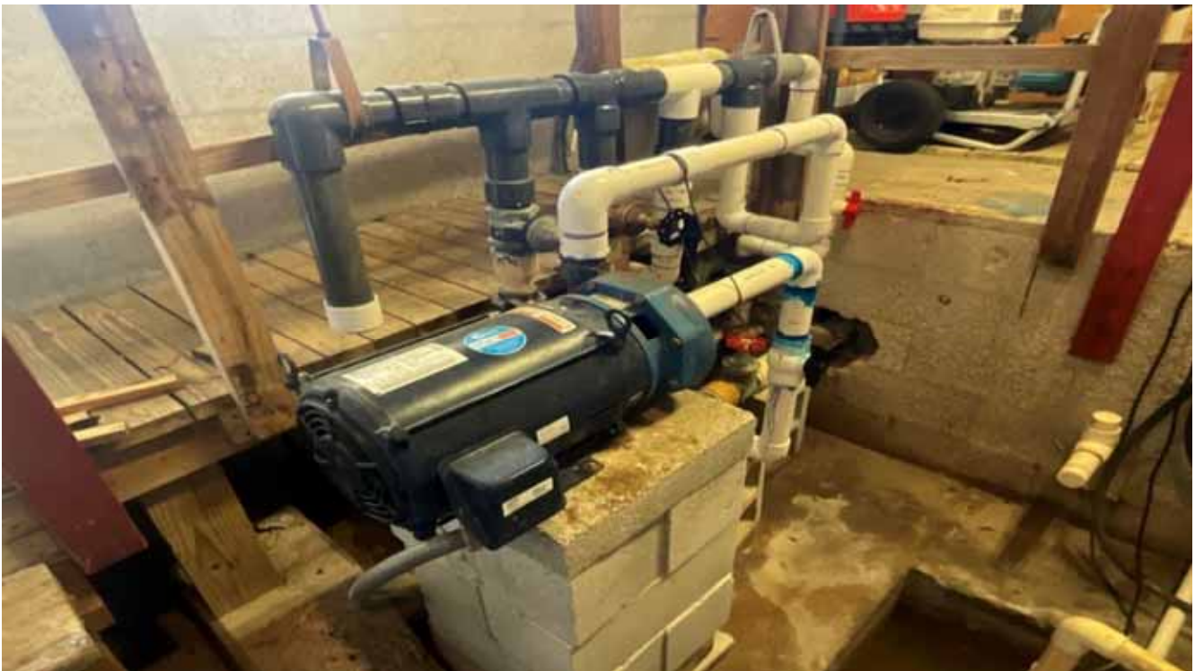
Irrigation Pump Equipment
