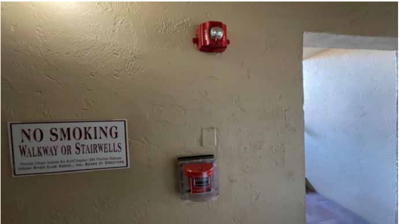
South Condo Bldg Fire Alarm System Devices
