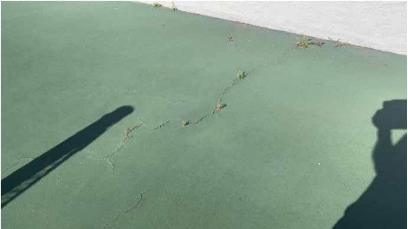
Tennis Court Surface Cracks
