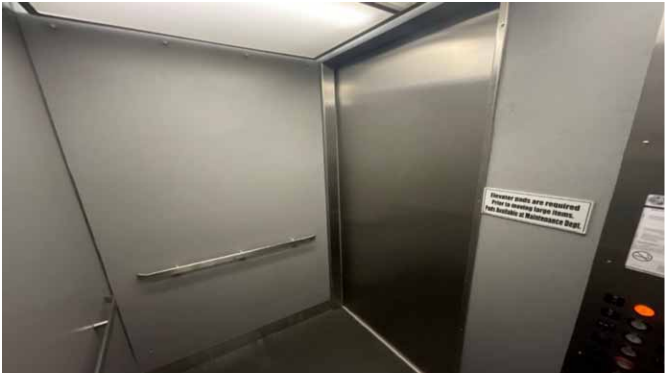
South Condo Bldg Elevator Cab
