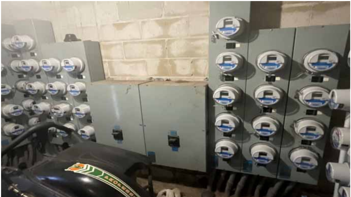
North Condo Bldg Electrical Panels
