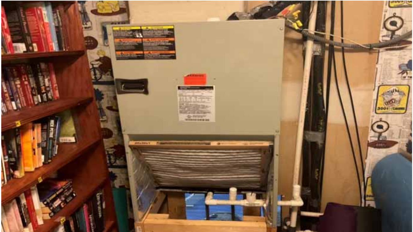
North Condo Bldg 4th Floor Fitness Rm AHU
