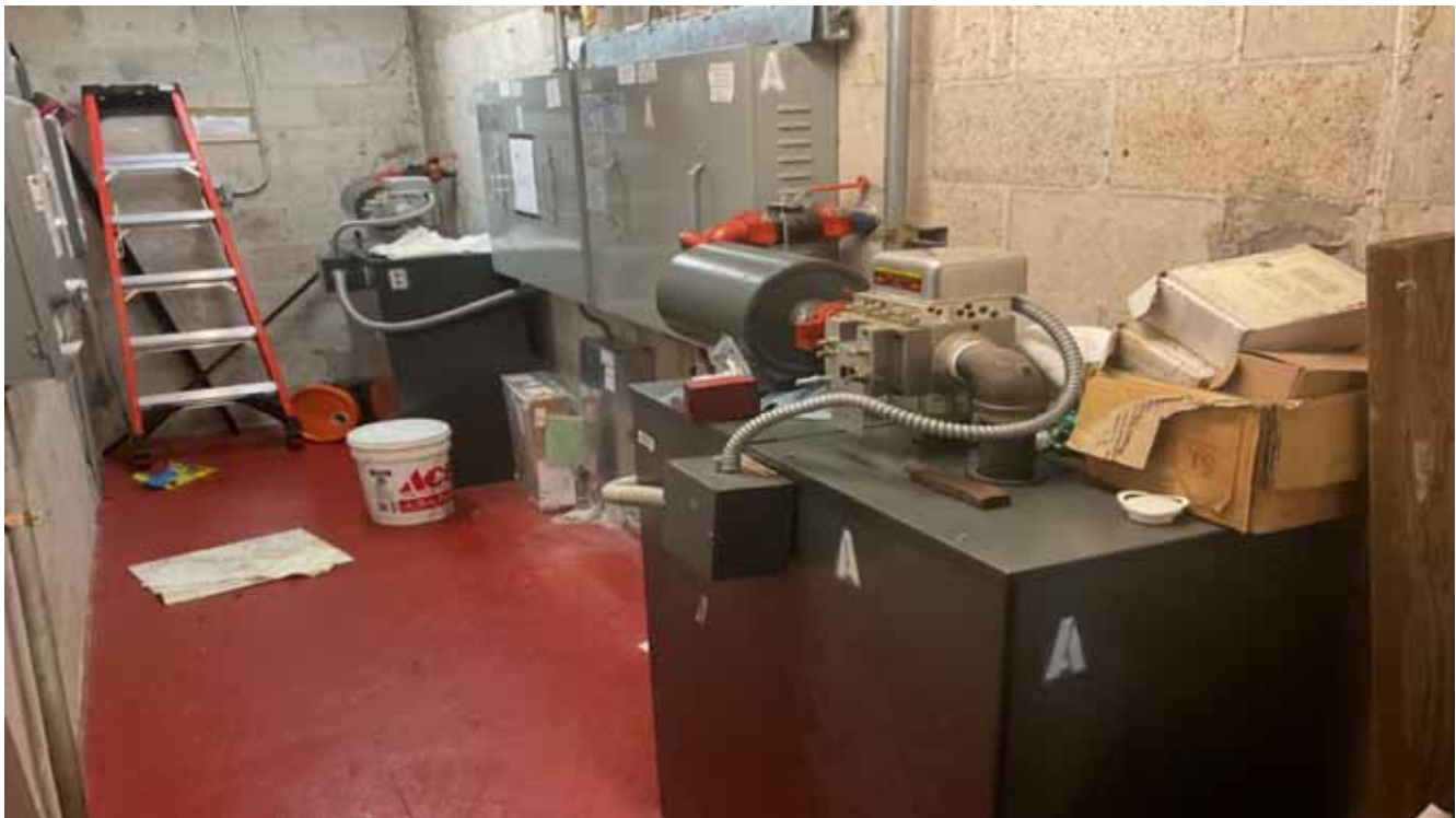
North Condo Bldg Elevator Equipment Rm
