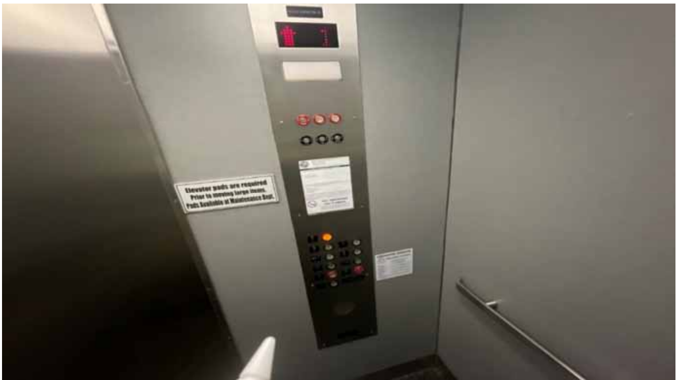
South Condo Bldg Elevator Cab
